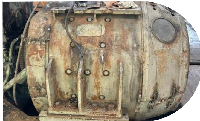
Main generator GP-312 (3 vnt.)
